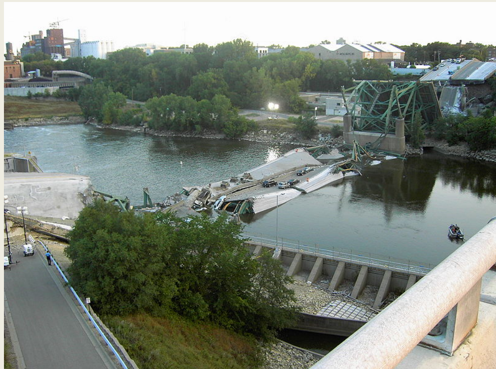
I-35W Bridge Collapse – Minneapolis, MN
